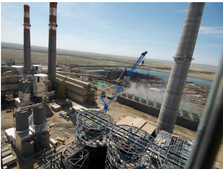
B&W's total-project scope includes design, procurement, construction and startup activities to facilitate the effective performance of the entire system and integration with existing or new emissions control equipment.
