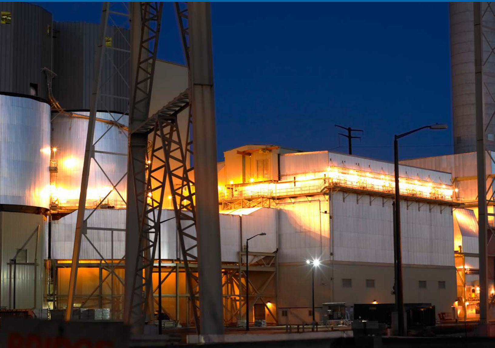
B&W PGG's SDAs and fabric filter provide an integrated SO 2 and particulate removal process.
