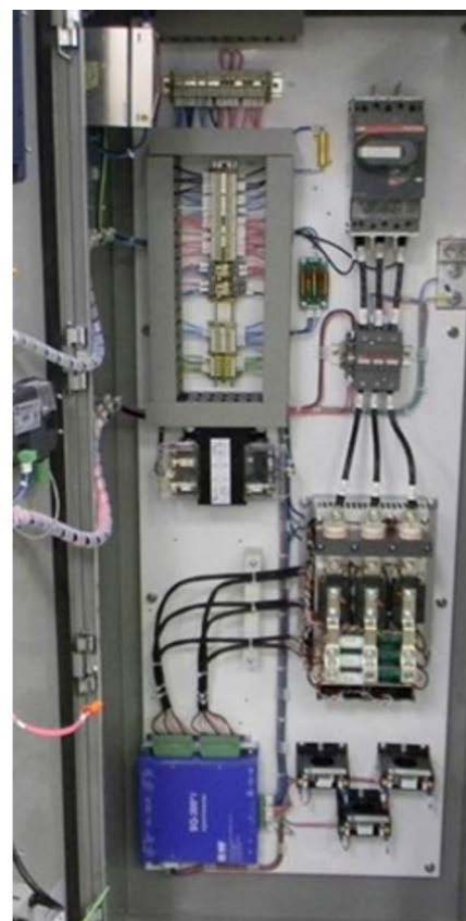
Typical three-phase AVC cabinet
