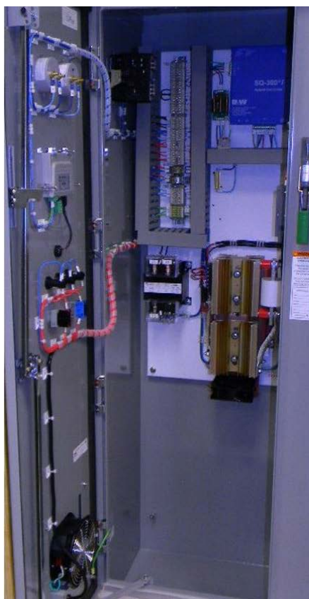
Typical single-phase AVC cabinet
