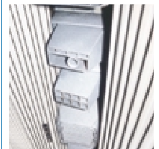
Coal and auxiliary air nozzles
