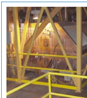
Separated overfire air ports
