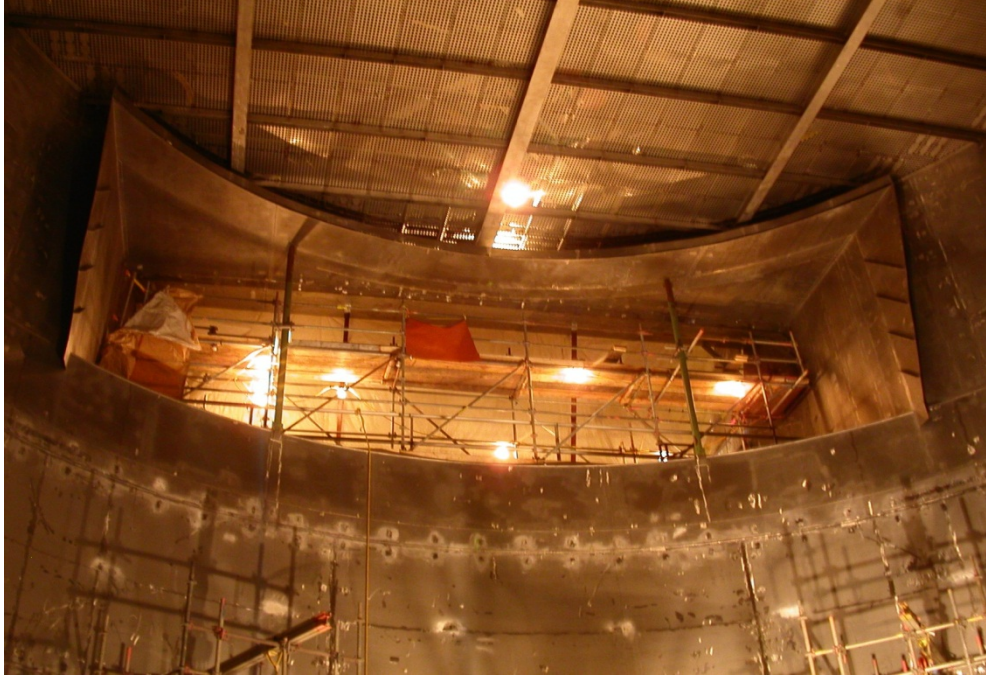
Figure 2: Interior of a spray tower retrofitted with a B&W tray
