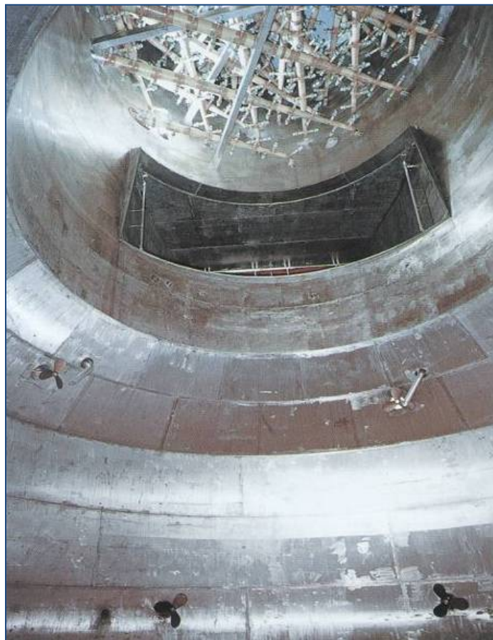
Figure 1: Interior of a spray tower (non-B&W) with no gas distribution devices.
