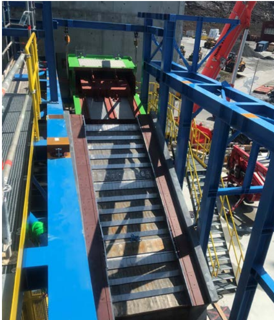
DynaGrate combustion grate and DynaFeeder fuel feeder system after lift-in.
